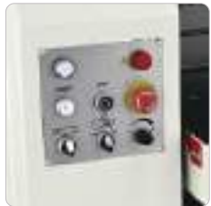
Electro-Mechanical Control Panel
